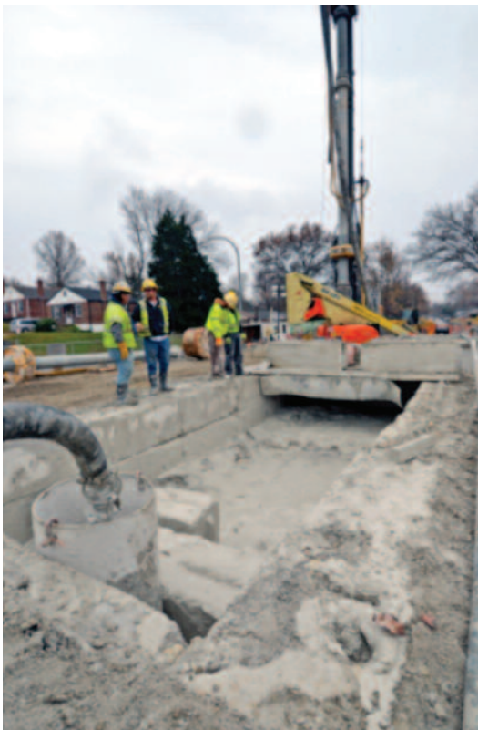
Temporary retention pool. Cuttings settle out to the bottom. Liquid is returned to the hole. The cuttings are periodically removed by a vac truck and hauled away to disposal off site.
