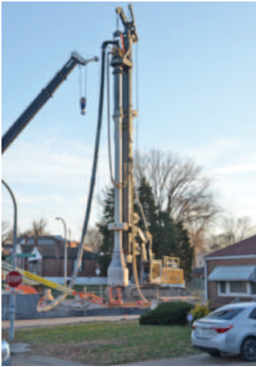
Tight spaces. A primary planning requirement of all MSD Project Clear phases is minimized impact on traffic and residents. The canister drilling method enables the crew to confine work to the median of a residential boulevard running perpendicular to this side street without detouring traffic.
